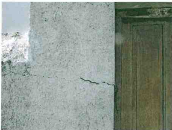
Boundary Wall needs repair
