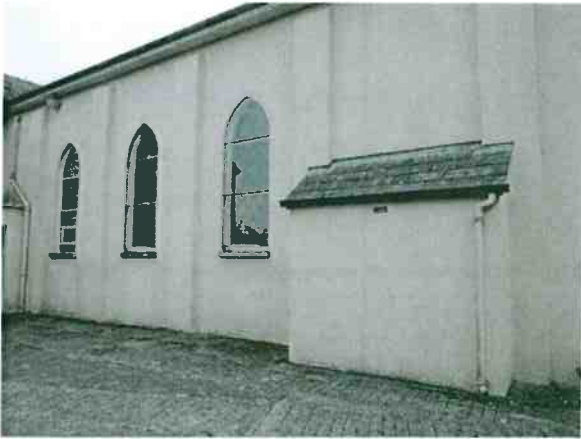
High Paving Level on North Side
