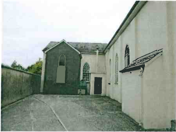
Visible Deflection in Roof of North Transept Slating Moderate Concrete Flat roofs may be uninsulated
