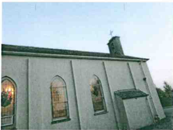
Slating looks poor on North slope
