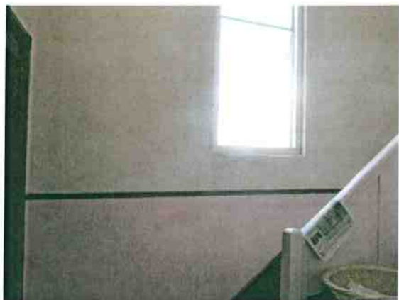
Poor window in Lobby/Stairwell
