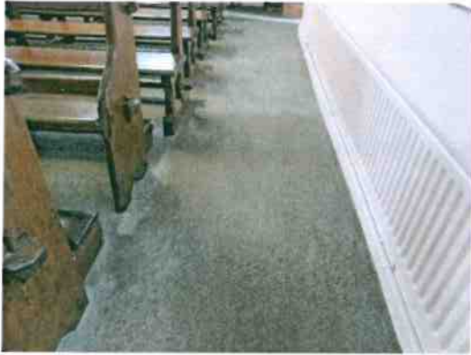
Floors could be damp under carpet
