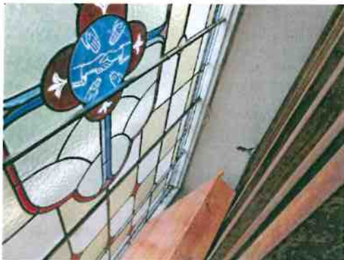
Stained glass needs cleaning Some frames need repairing and replacing Storm glazing needs to be considered
