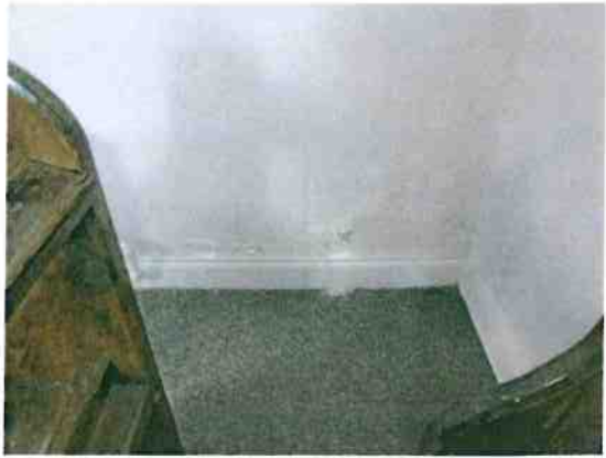
Dampness in walls
