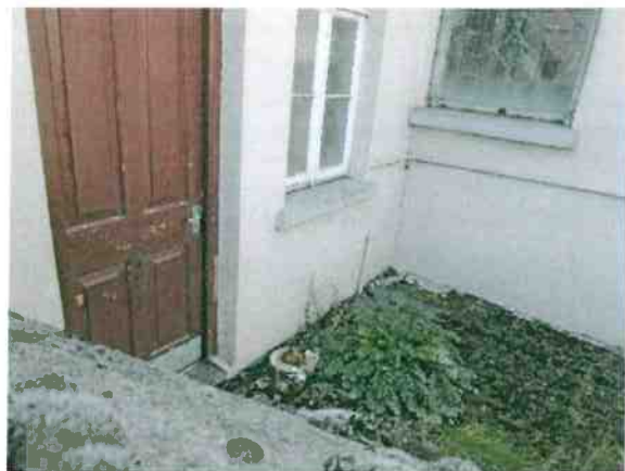
External doorset to Sacristy poor Yard needs to be cleaned and surfaced
