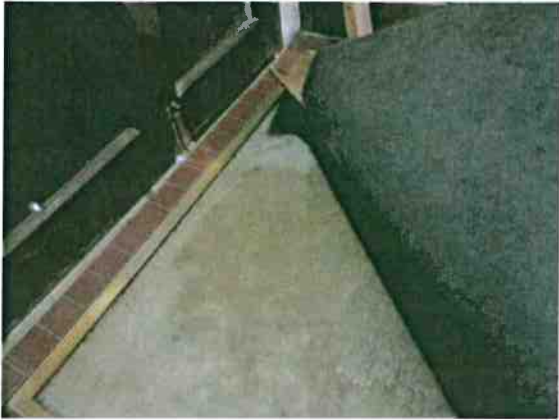
Front Door in poor condition Rain getting in also
